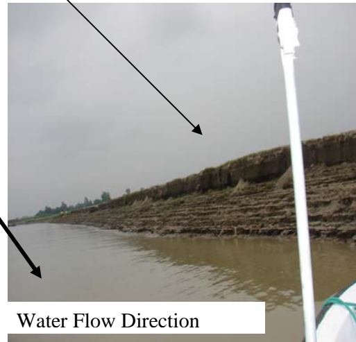
Figure-4b: Eroding unstable river bank before bandals construction
